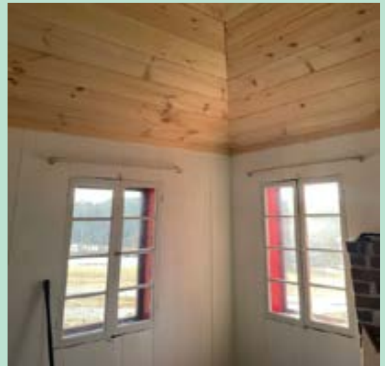
Inside Edgewood - new cathedral ceiling will allow for a fan (photo by Liz Ryan Cole)
